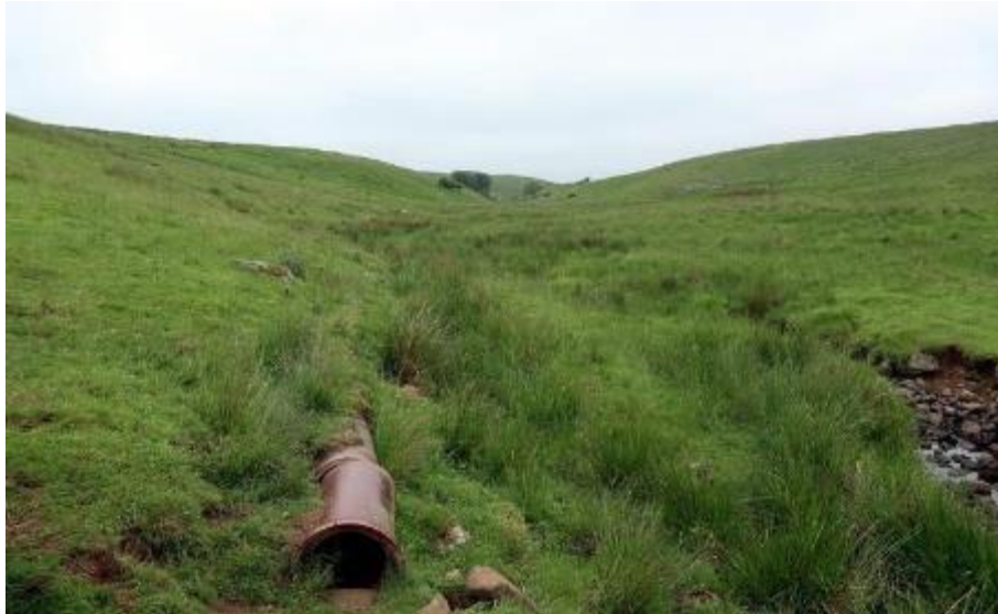
Exposed ceramic pipeline (P20, 2022 Report)
